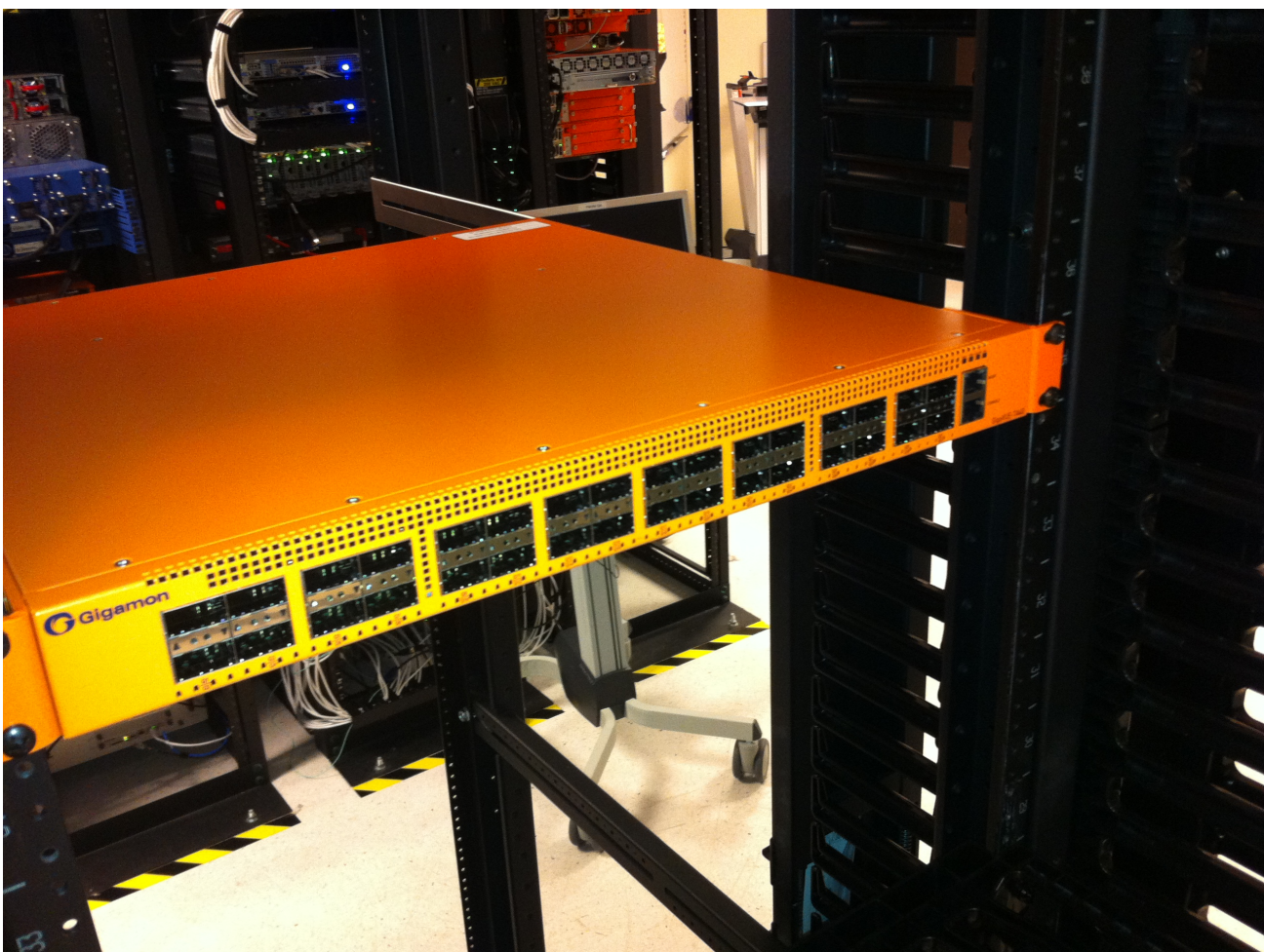
Figure 12 Front View of the Mounted Node to the Four-Post Rack
