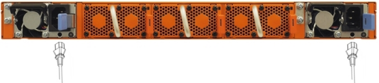
Figure 17 Connecting AC Power on a GigaVUE TA Series-TA100
