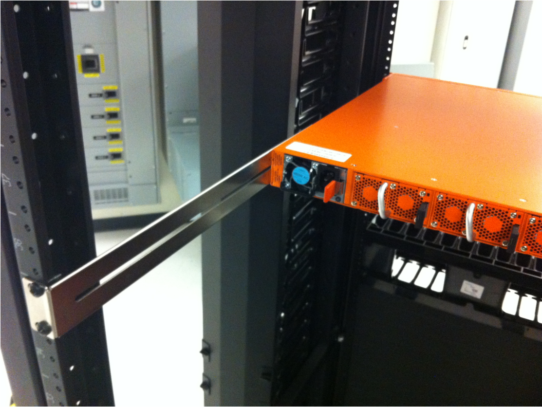
Figure 13 Rear View of the Mounted Node and Rails on the Four-Post Rack
